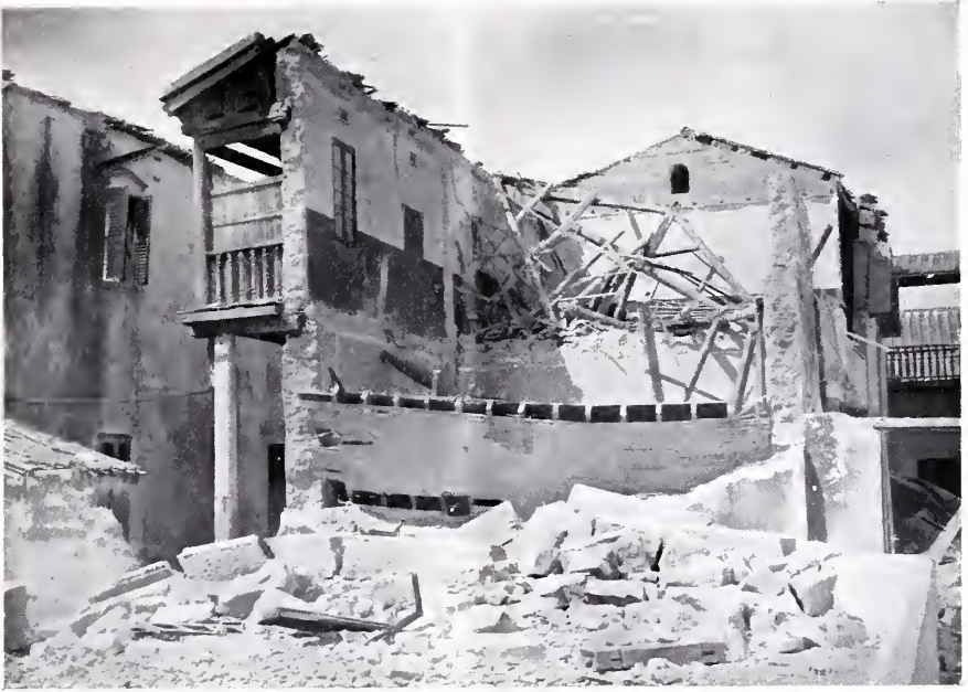
CHAOCHOWFU HOSPITAL AFTER EARTHQUAKE.
